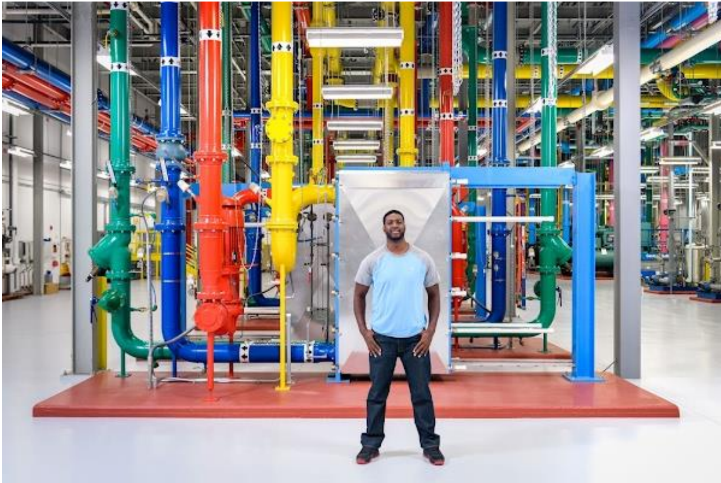
Google data center
